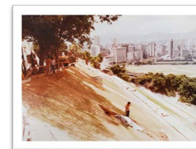
Slope maintenance works at the Hong Kong Sanatorium adjacent to the Happy Valley Racecourse (1977) (Reference no.: HKRS2118-4-1)
